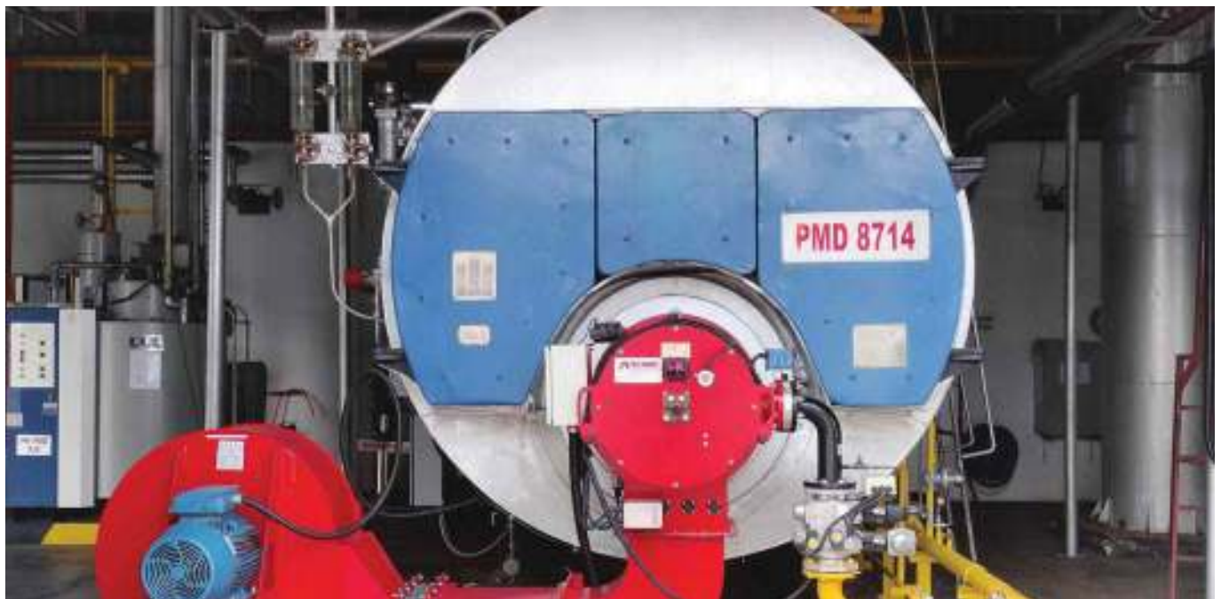
Boiler in Ipoh Plant
