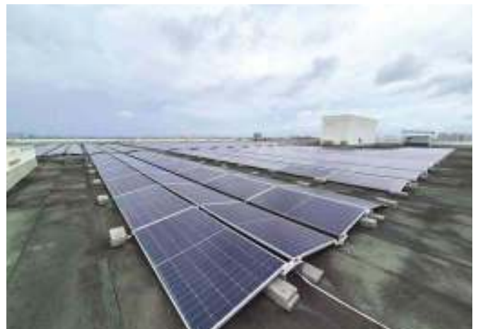
Solar photovoltaic panels in Singapore plant
